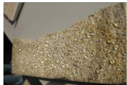
Condition on rough masonry surface
